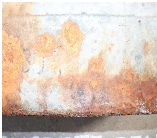
Beam specimen after accelerated corrosion
